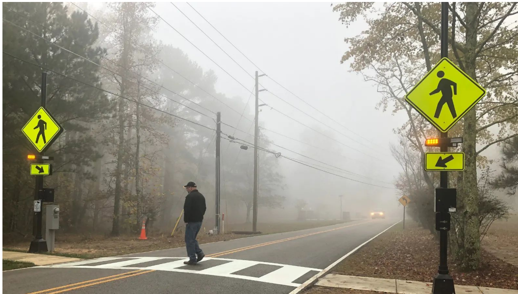
Rapid Rectangular Flashing Beacon (RRFB)
